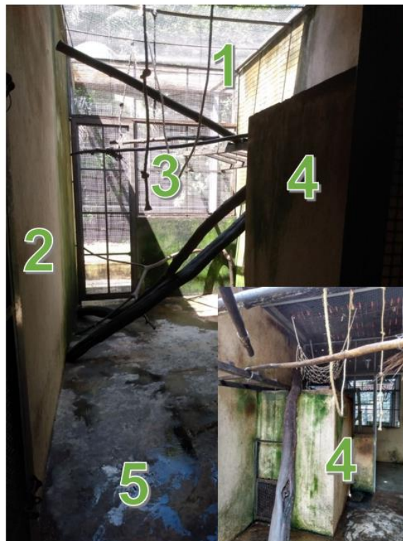
Figure 2.3. Front (large) and back (small) views of enclosures C, D, E and F. (1) Metallic mesh ceiling, (2) concrete side wall, (3) back wall made of metallic mesh and concrete, (4) concrete inner cage (entrance seen in the small picture) and (5) concrete floor. Environmental enrichment structures can also be seen.
