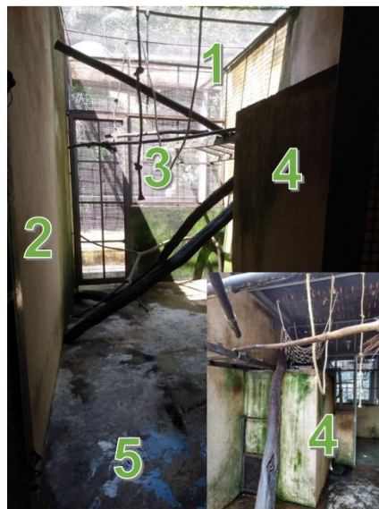
Figure 4.2. Front (large) and back (small) views of enclosures C, D, E and F. (1) Metallic mesh ceiling, (2) concrete side wall, (3) back wall made of metallic mesh and concrete, (4) concrete inner cage (entrance seen in the small picture) and (5) concrete floor. Environmental enrichment structures can also be seen.
