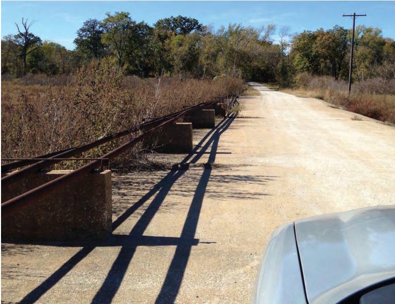
Figure 18.1: Minimal expenditure on pipeline safety. Oil pipelines at Hagerman National Wildlife Refuge, Grayson County, Texas, US. In wetter weather, water routinely flows over this road while large tree trunks float down the stream that floods this area. Photographer: Peter C. Schulze.
