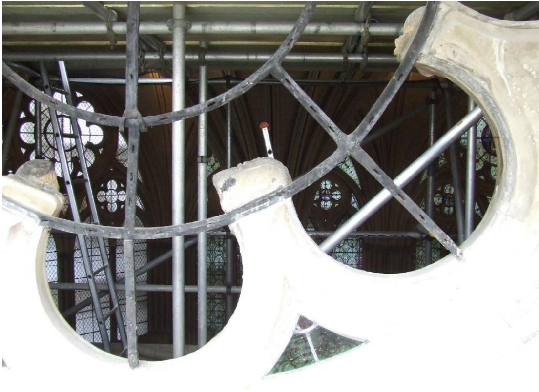
Figure 5: Metal work set up ready to receive the glass at the Chapter House, Salisbury Cathedral. Photo: Sam Kelly
