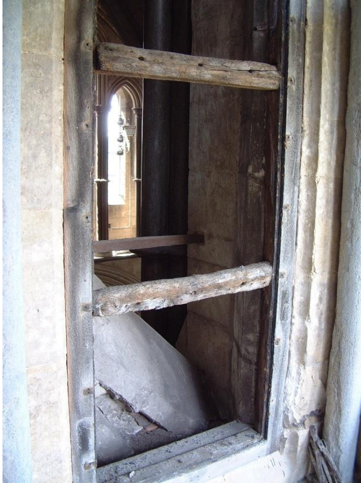
Figure 3: Medieval timber window frame at Salisbury Cathedral. This has a cover strip over \frac{3}{4} of the frame that is 19th century and forms a rebate. Photo: Sam Kelly
