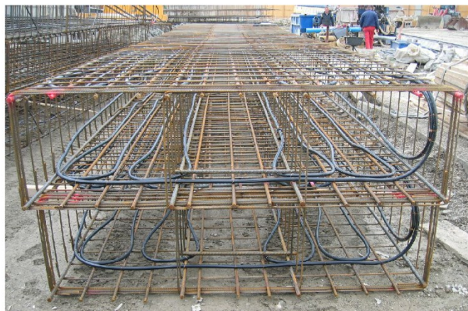
Figure 2-20: Reinforcement cage with heat exchanger pipes for thermo-active diaphragm wall (Hofinger & Kohlböck, 2005)
