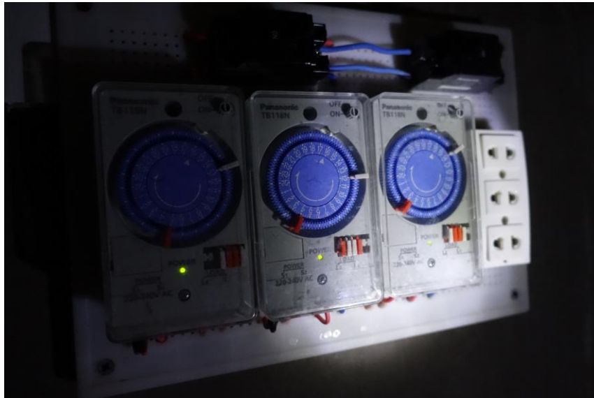
Figure 12 Timers for switching daytime and nighttime
