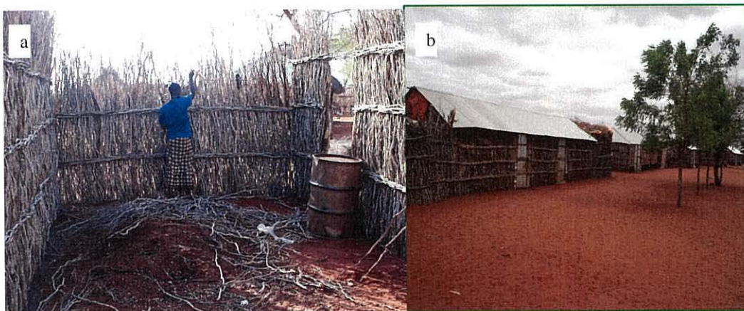
Plate 3.3 a) Man constructing a house, b) homes built from Cordeauxia edulis wood at Gambare village, Ogaden, Ethiopia (Photo by: Mussa. M. Yusuf)
