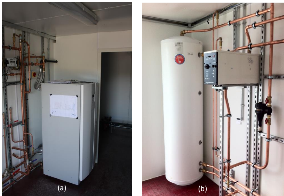
Figure 45. (a) Heat pump. (b) Buffer tank.
