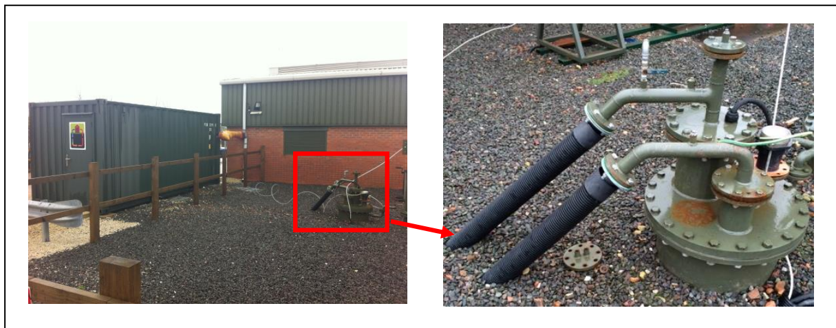
Figure 43. Mine water flow and return pipe.
