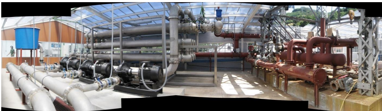
Figure 58. Heat exchanger in Barredo Shaft (left)
