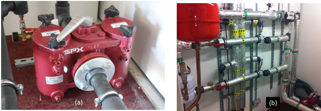
Figure 44. (a) Filter. (b) Heat exchanger.
