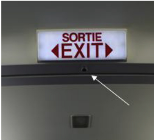
Fig. 2. Position of a temperature/humidity sensor in the ceiling of the cabin.
