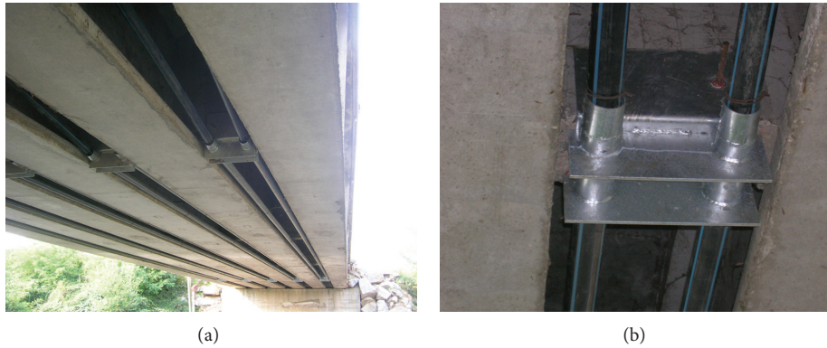
FIGURE 5: (a) View of external prestressing; (b) metallic saddle of deviation.
