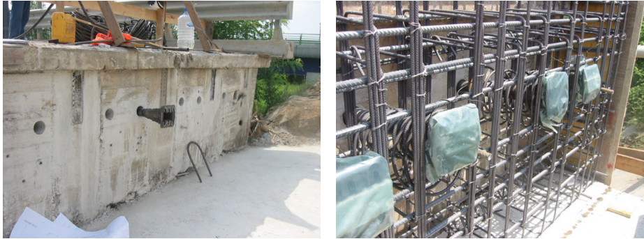
FIGURE 4: Anchor heads and antispalling reinforcement.
