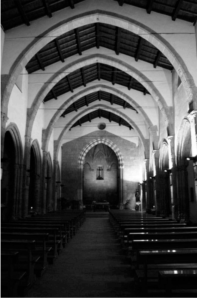
FIG. 1. Diaphragm arches and wooden ceilings in the church of San Francesco in Iglesias (photo by author).
