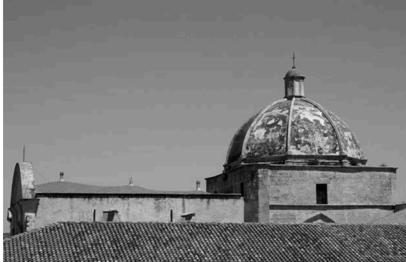
FIG. 10. View of the extrados of the vaults and the dome of the Jesuit church in Sassari (photo by author).
