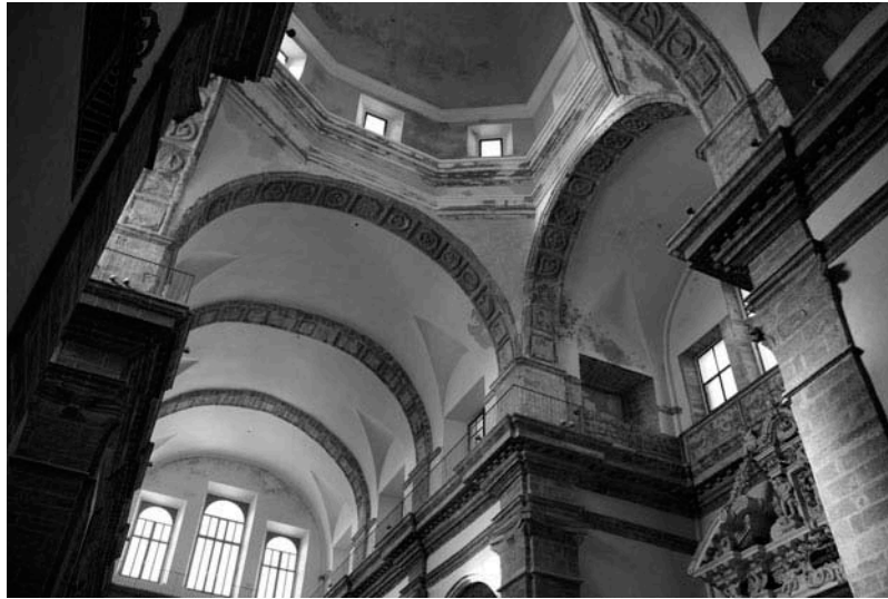
FIG. 19. View of the vaults and the dome in the church of S. Michele in Alghero.
