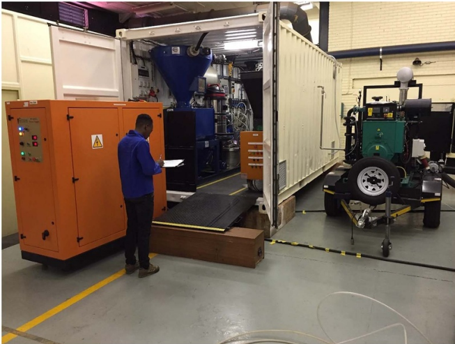
Figure 29. Containerized plasma waste to energy system.
