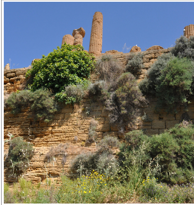
Figure 10 - Portion of the ridge characterized by dense bushes; in this area the ridge is largely consolidated with a masonry block wall.
