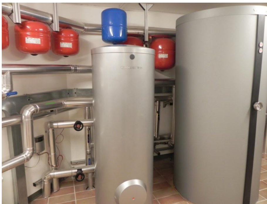
Figure 29 Images of the Auxiliary boiler
