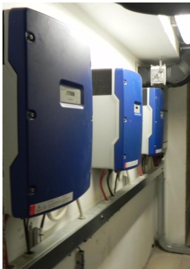
Figure 30 The DC/AC photovoltaic converters
