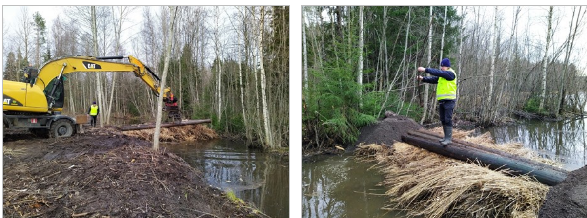
Figure 3. Construction of the common reed filter (left) and measurement of the dimensions of the new filter (right) in November 2020. The filter consisted of common reed bundles with logs on top of them. Photos: M. Vahvaselkä.
