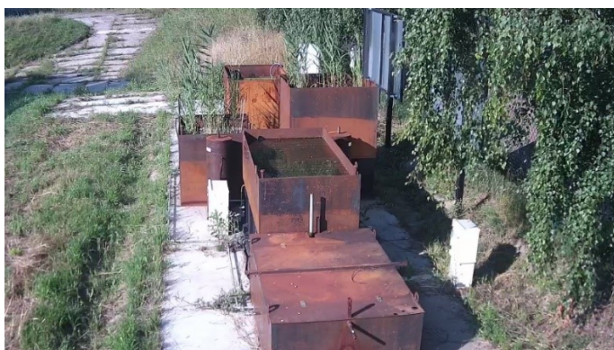
Figure 17. Pilot station for the stormwater treatment. Photo: GW.
