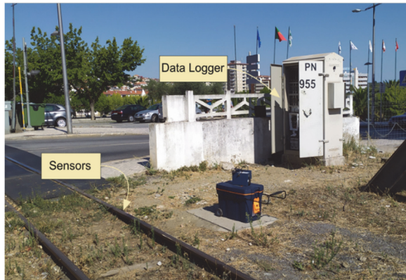
Fig. 3 – Sensors of the rail.
