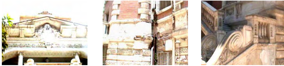
Fig.9 deteriorated parts due to the moisture and atmospheric effect.
