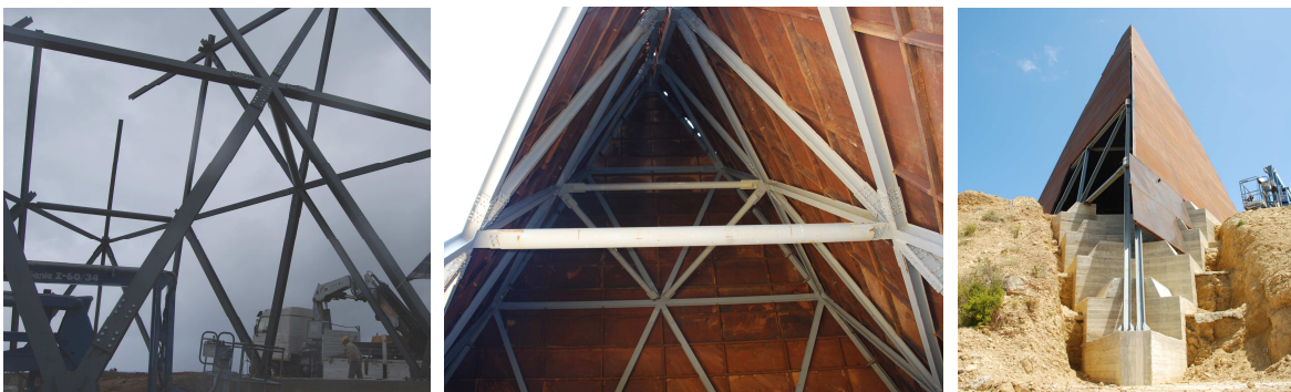
Figure 9: Construction works. 3D steel alveolar structure assembling. COR-TEN sheets assembling. View from above.
