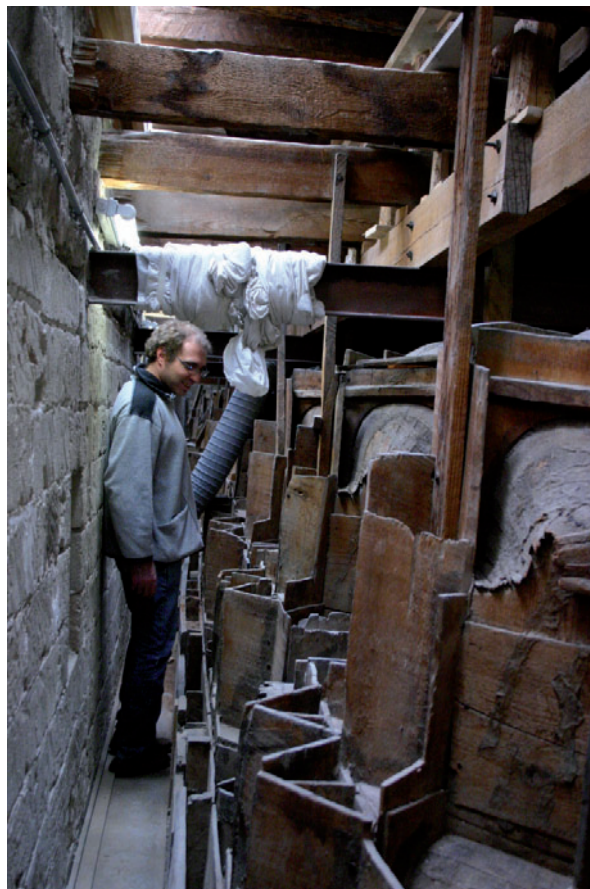
Fig. 59. The extrados of the ceiling. (Photo: courtesy of Arch. Mario Li Castri)
