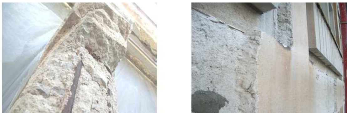
Figures 4 e 5. Lack of plaster (left) superficial deposits with yellow patina (right)
