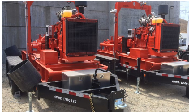
Portable pumps at the Diablo Canyon NPP ready for deployment.
