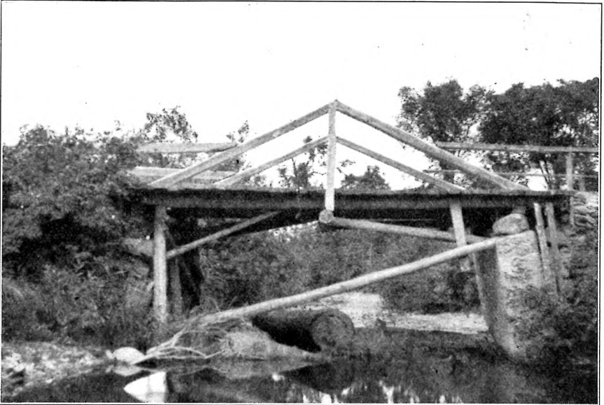
Bridge abutments in unsatisfactory condition for service. Deformed by frost action and stream scour. Right abutment "jacketed" with concrete intended to prevent the collapse of its original breast wall.
