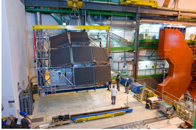
Figure 3.13: View of the seven modules of the HMPID mounted on the cradle.
