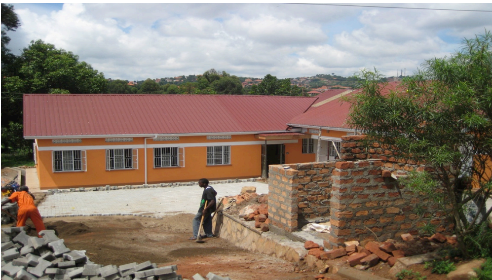
Figure 14: Renovation of Ggaba outreach clinic for decentralization of HIV/TB services into the communities (work-in-progress)
