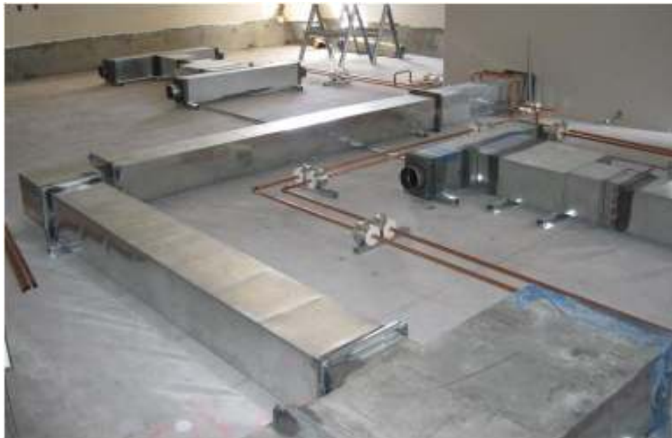
Figure 2-2 Real case ductwork
