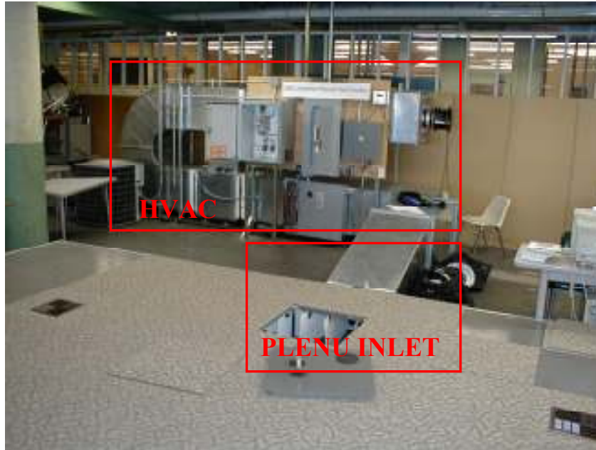
Figure 4-5 Plenum facility HVAC system and underfloor plenum
