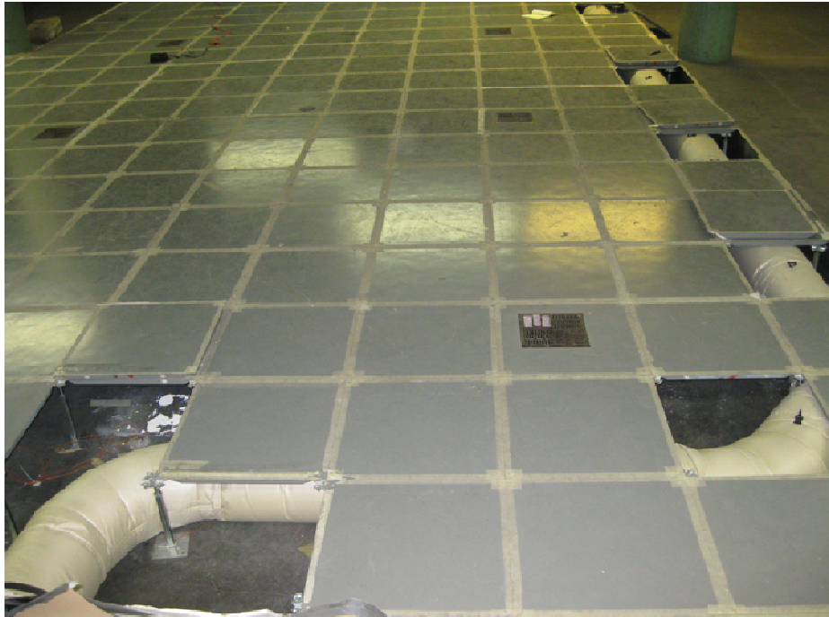
Figure 2-3 Fabric duct in underfloor plenum
