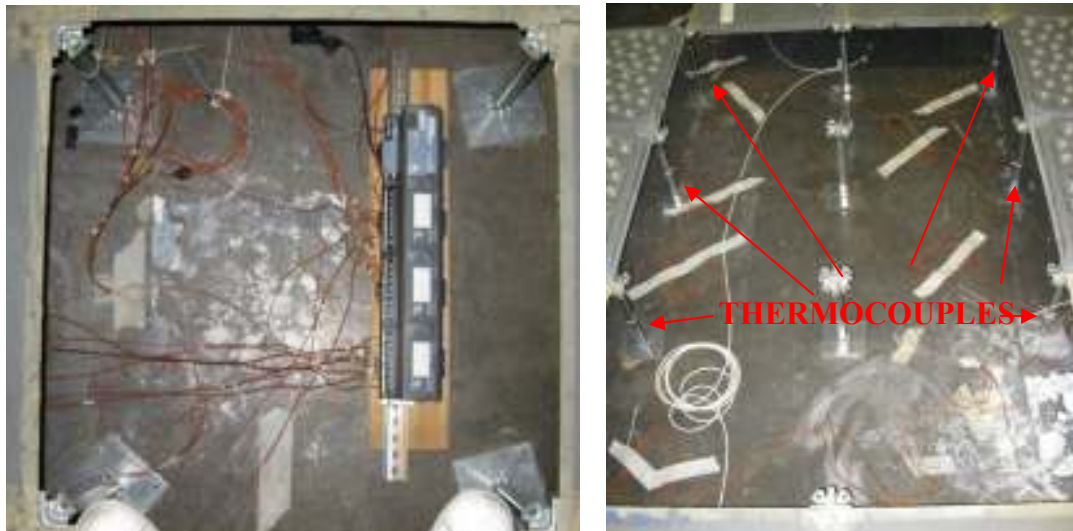
Figure 4-6 Data acquisition system and thermocouples inside the plenum
