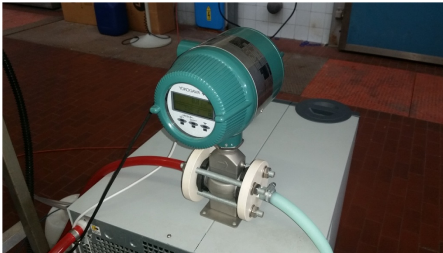
Fig. 5.31 Water flow meter
