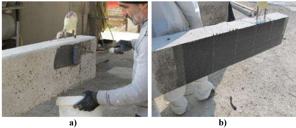
Figure 3-5 FRP strengthening procedure: a) application of first resin layer; b) FRP-strengthened beam
