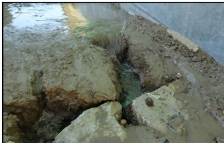
Figure 3.14. Section showing the holes just upstream of the wall in the first preparatory tests
