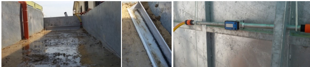
Figure 3.7. The spillway located upslope and feeding the hillslope behind the stone wall
