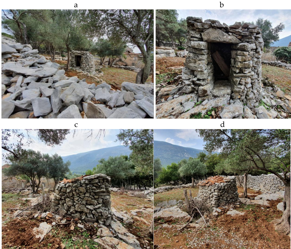
Figure 102. A dry stone water closet, part of one of the buildings in Veli Tržić (a-d), partially covered with stone slabs and roofing tiles (2021)
