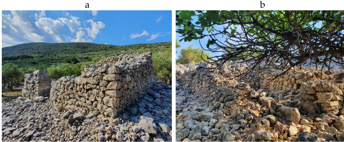
Figure 91. The common current state of many field huts: a) Roof collapsing as the first stage of degradation. b) In an advanced stage of degradation, one of the last indicators of its use is the interior niche (2020)
