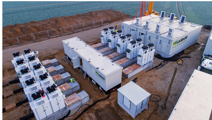
Figure 3: Leclanché Storage Power Plant in Graciosa
