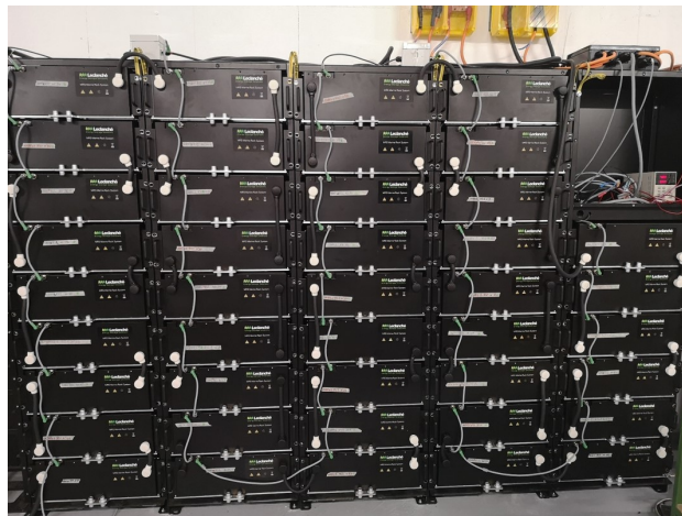
Figure 59: Marine Rack System (MRS)
