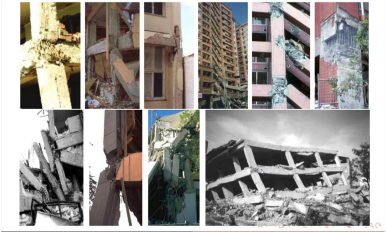
Fig: 1.1.2: Failure of Structure due to Shear Failure of the Joints ( Ref: webinar by Ben Deaton )
