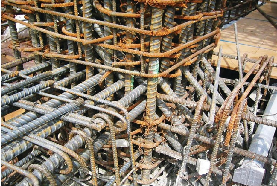
Fig. 1.1.5: Congestion at the Beam-Column Joints ( ref.: www.concreteconstruction.net )
