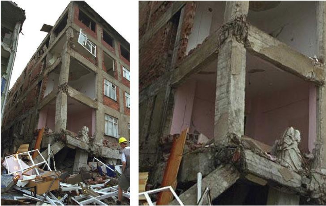
Fig. 1.1.3 Damage in the exterior joints Kacholi earthquake, 1999 (Ref: webinar by Ben Deaton)
