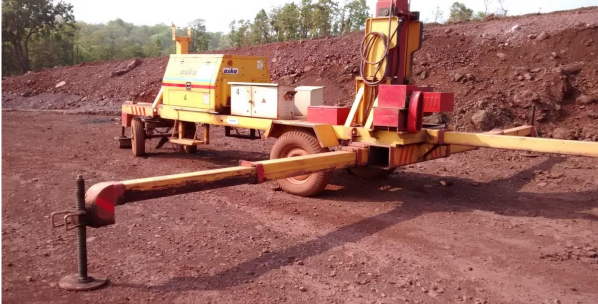
Figure3.2 Diesel Generator set in an iron ore mine
