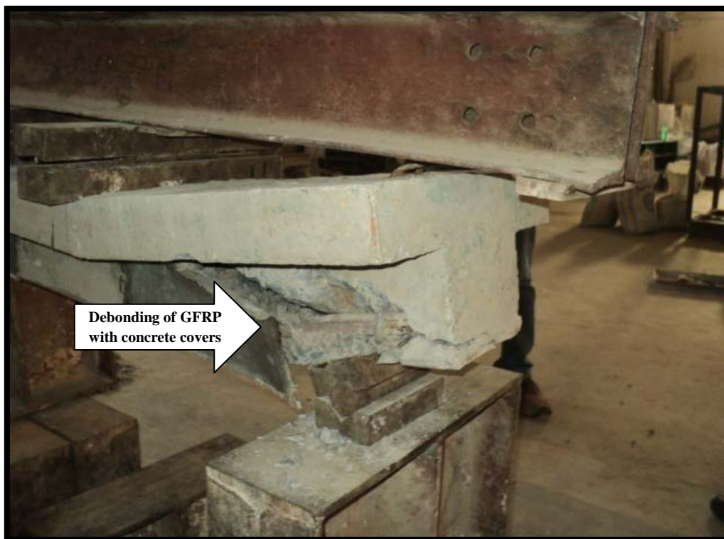
(c) Shear failure of beam -Debonding of GFRP sheet
