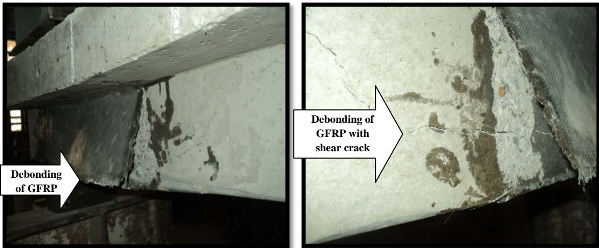
(b) Debonding of GFRP sheet followed by shear failure
