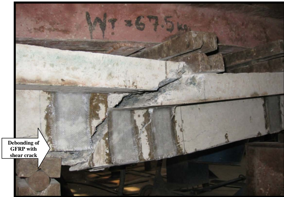
(c) Debonding of GFRP sheet followed by shear failure
