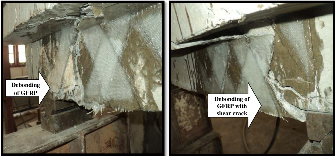
(b) Debonding of GFRP sheet followed by shear failure
