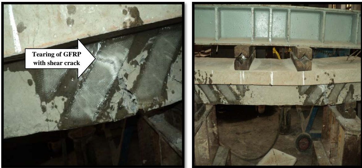
(c) Tearing of GFRP sheet followed by shear failure
