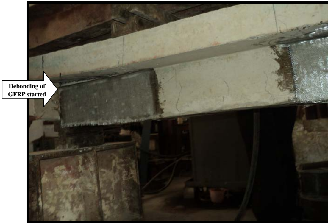
(b) Initiation of debonding of GFRP sheet
