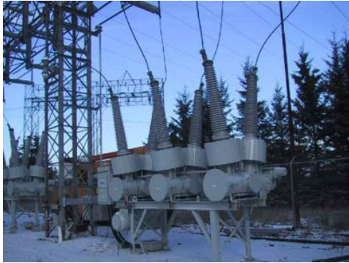
Figure 3.4 1200 A, 3-pole 115,000 V Breaker at a generating station
