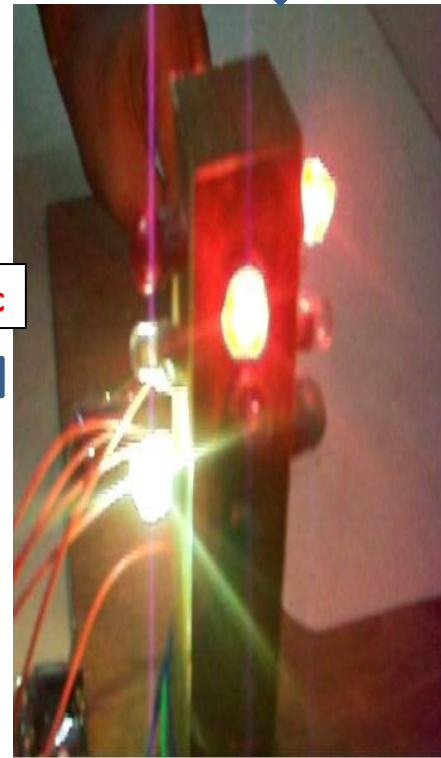
Green light ON of lane 1 (Emergency status ON)
