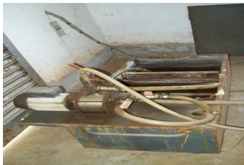
Fig no. 3.2.3.1 Electrolyte tank
