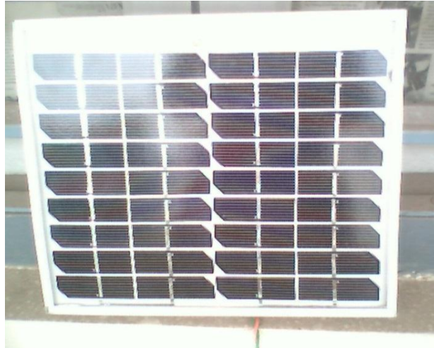
FIGURE 4.3: PHOTOGRAPH OF THE SOLAR ARRAY
