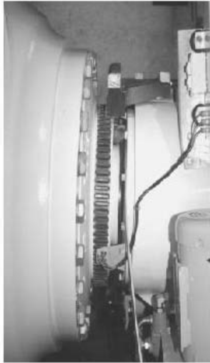
Figure 10: Low-speed Shaft speed Sensing System
