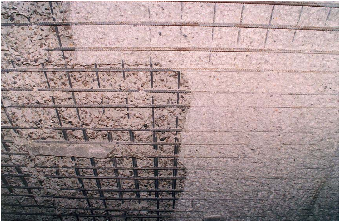
Fig 1.1: fire damaged slab
