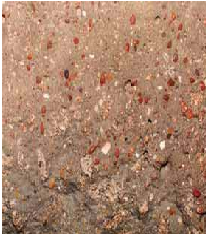
Fig 1.4: Color change in the concrete due to elevated temperature
