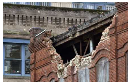
Fig 1.2 Parapet failure (Non-structural failure)
