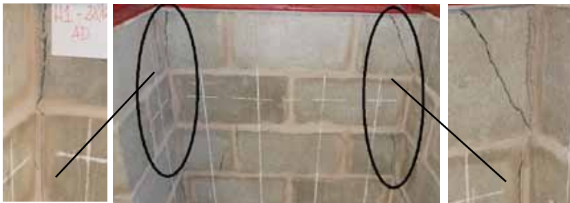
Figure 9 — Failure mode of specimen.
