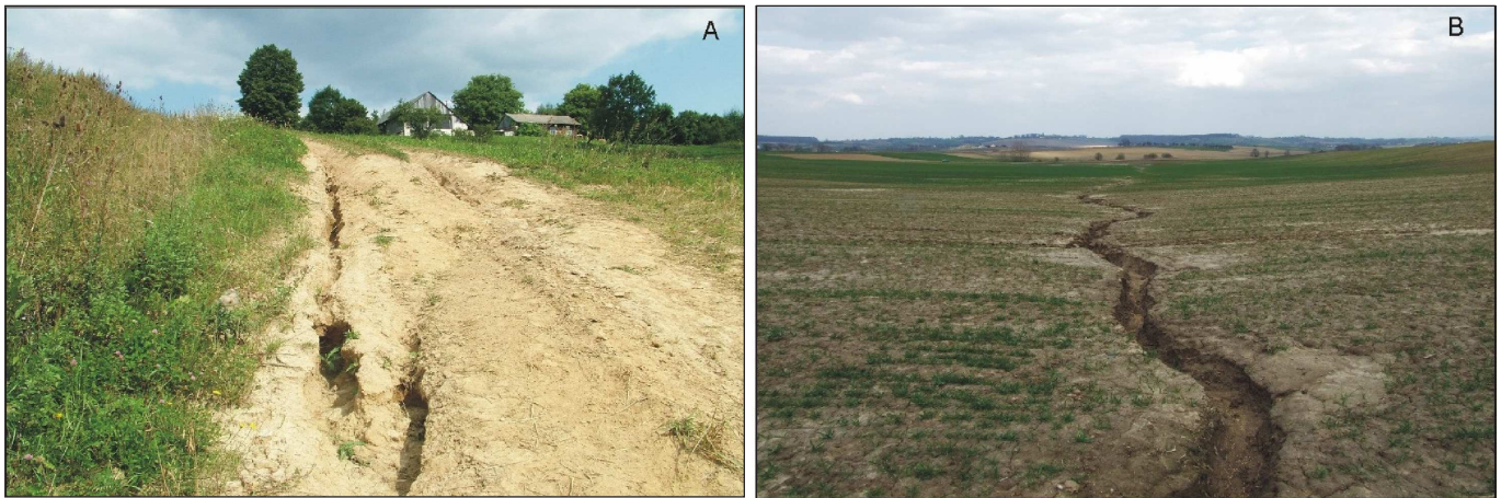
Figure 8. Development of gullies along the cart roads (A) and natural drainage lines (B) in Wieliczka Foothills (photo J. Swiechowicz)
