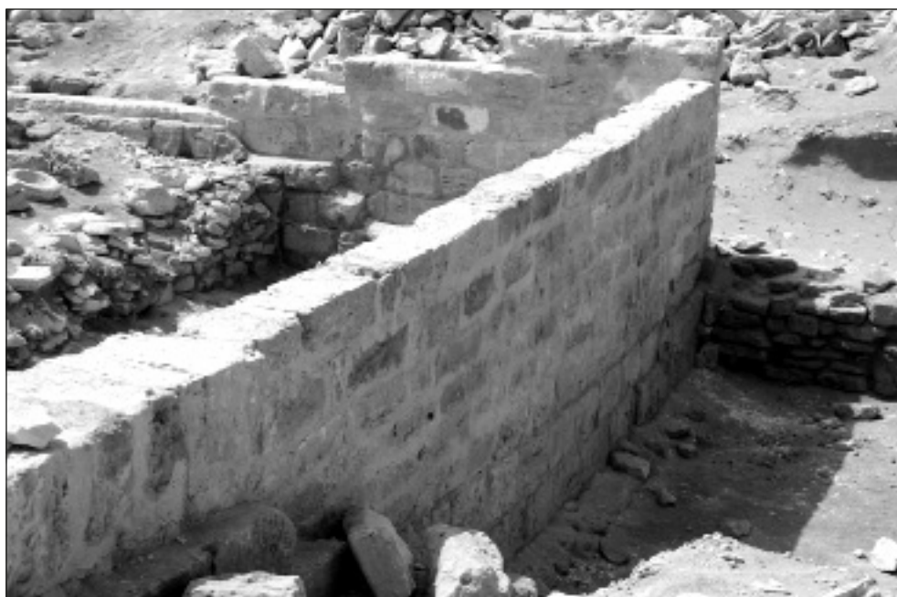
Fig. 2. House 1, southwestern corner before (top) and after conservation in 2008, view from the northwest (Photo P. Zambrzycki)
