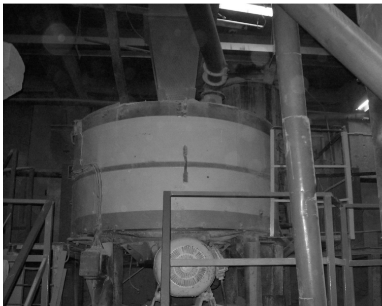
Photo 1. Devices operating in an environment heavily dusted with ore
