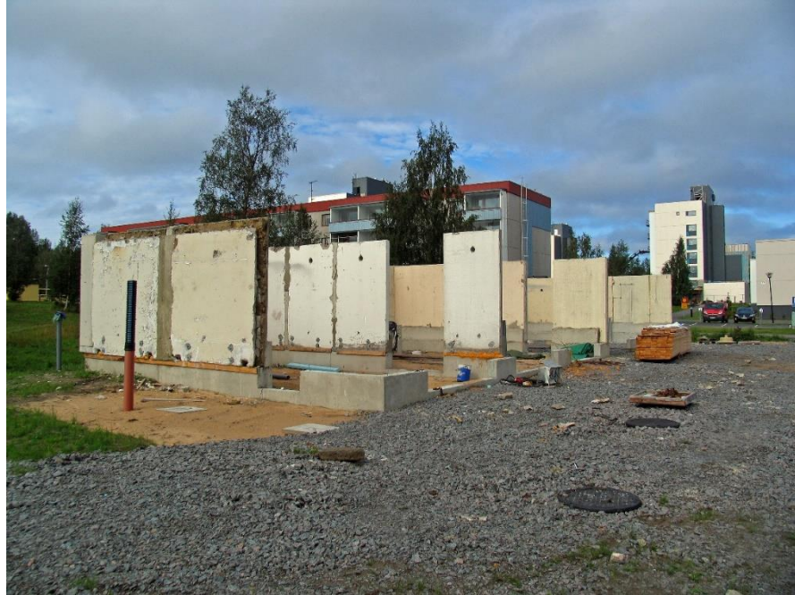
Figure 12: Construction of the maintenance building from reused components in Kummatti, Raahé. In the distance, a partially deconstructed finished building can be seen. (Photo provided by an interviewee)
