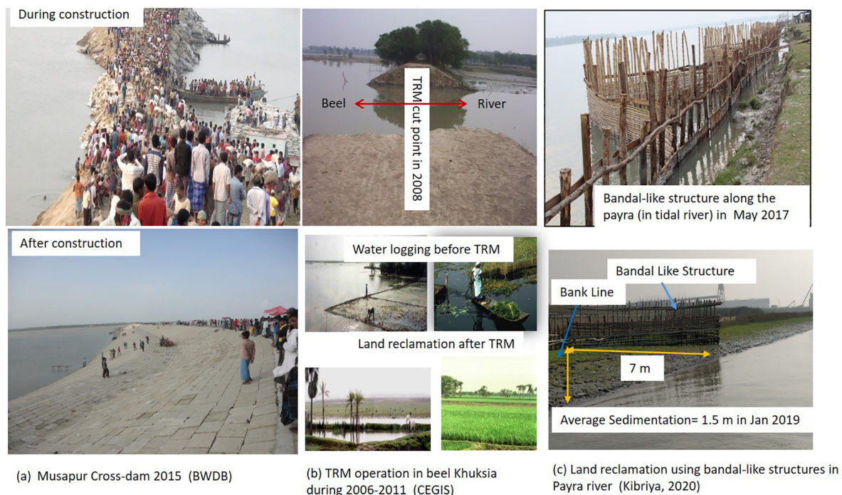
Fig. 6. Field examples of cross-dam (left), TRM (middle) and bandal-like structures (right) as practiced in Bangladesh's coastal zone. Cross-dams are a labor-intensive construction as it needs to utilize the specific tidal phase to construct the main barrier (left-top photo) and later transforms into a permanent structure (left-bottom photo). For TRM, the man-made canal connects the river with the beel (middle-top photo). Due to TRM operation, the natural dredging of the river solves the waterlogging problem (middle-mid photo) and at the same time, fills the beel with sediments causing building of new land (middle-bottom photo). Bandal-like structures are made with eco-friendly soft materials (right-top photo) to stabilize the riverbank with reclaimed land and increase the conveyance capacity of the river (right-bottom photo).
