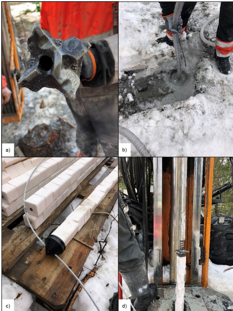
Figure 3. a) 90 mm drill bit used for pre-drilling. b) 32 mm reinforced hose for pumping KCl slurry into the pre-drilled borehole. c) KCl poles in 1 m sections ready for installation. d) Installation of KCl poles.
