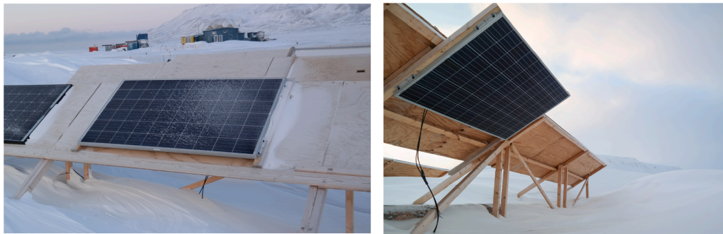
Fig. 2. Module installation with a sky-facing module (left) and a ground-facing module (right). The modules are lifted 2 cm from the wooden surface to allow for ventilation on the backside.
