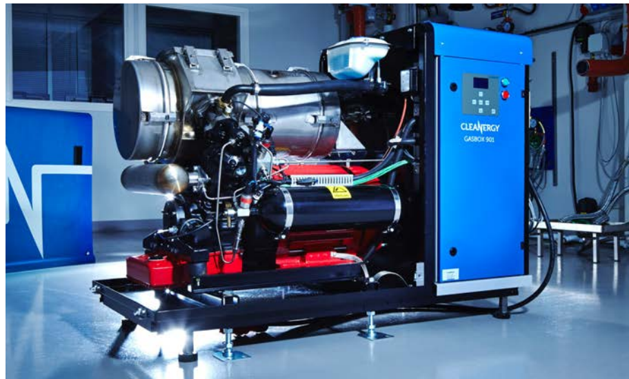
Figure 6-26: CHP Stirling engines (PU BU 1.3) produces heat and electric energy
