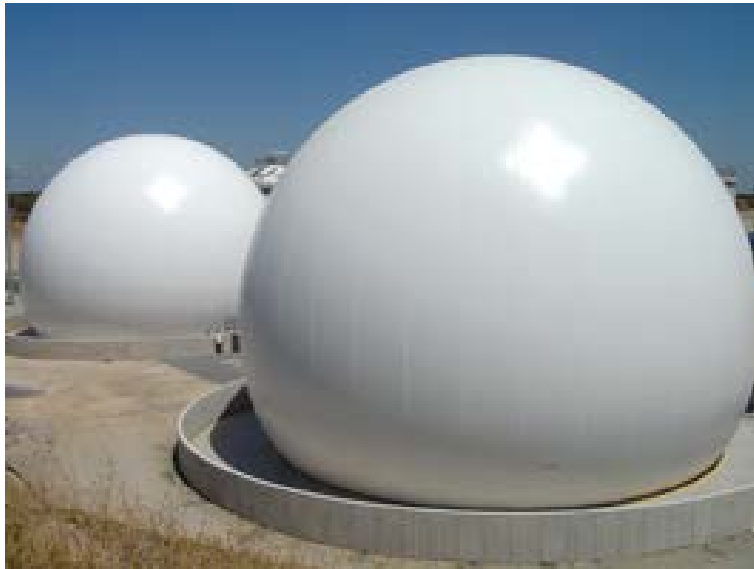
Figure 6-23: stand-alone vessel (BP GS 2.2) is external to digester to compensates biogas
