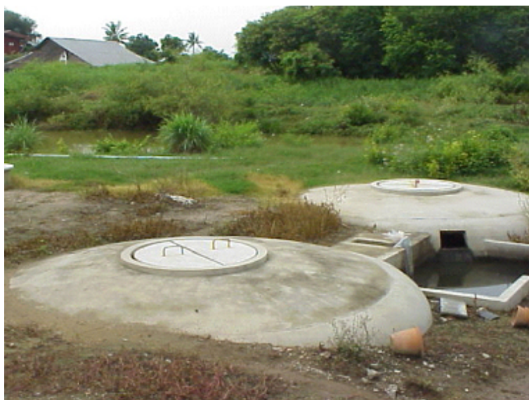
Figure 6-21: fixed-dome reactor (BP DR 1.2) has constant volume, usually is an underground digester that has minimal temperature exploiting ground insulation. Made of concrete and buried, it has a long-life span
