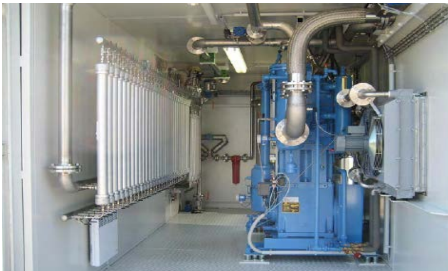
Figure 6-28: scrubbing technology (PUBU 1.9)
