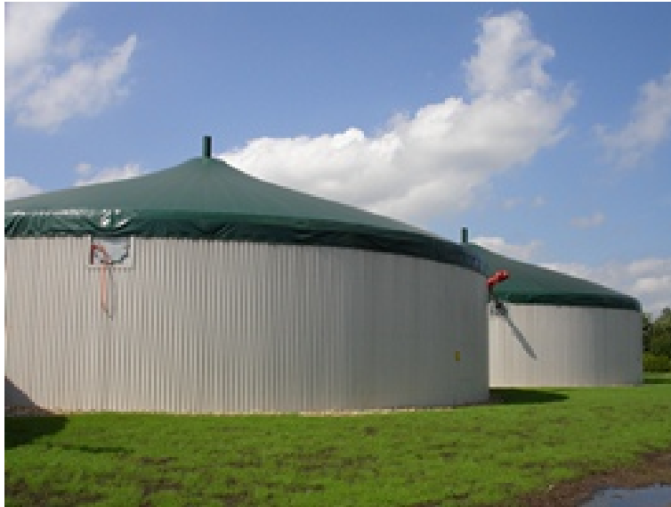
Figure 6-22: floating-drum reactor (BP DR 1.3) with integrated gas storage (roof double-layer BP GS 2.1). Reactor has expandable a volume that compensates biogas fluctuations
