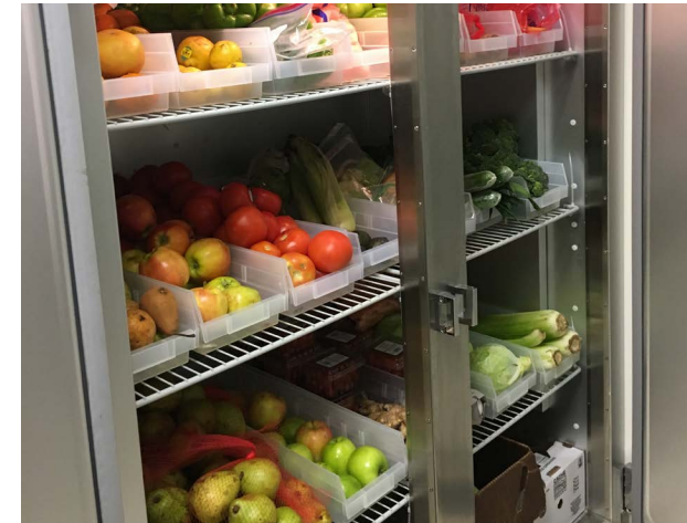
Community Kitchen - Example of Commercial Cold Storage Unit at Providence Milwaukie's Community Kitchen
