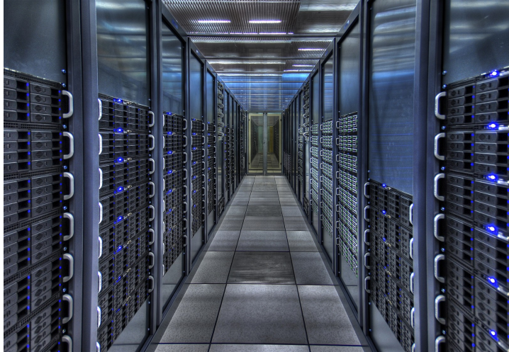
Figure 1.15: The CERN Data Centre.
